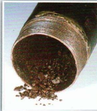
High humidity - Rusty pipeline
